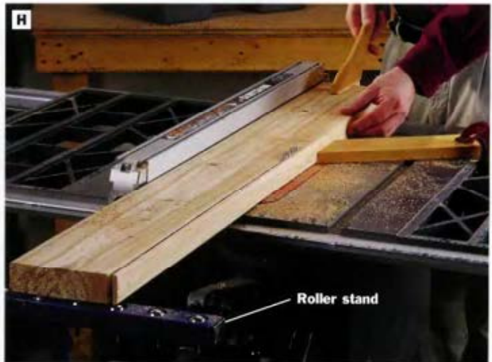
PHOTO H: Rip-cut 2 × 6 stock down to a width of 5½ in. to form the tabletop slats. You could make these cuts with a circular saw and straightedge guide, but a better choice is to use the table saw and rip fence. Support workpieces with a roller stand as they leave the saw table.
