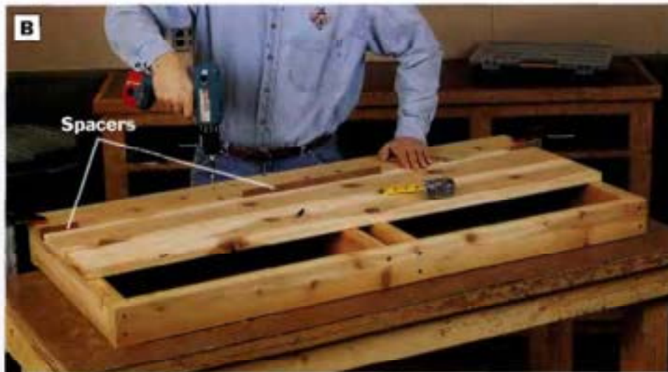
PHOTO B: Install the seat slats on the bench seat frame with screws. Position the back seat slat 7 in. from the back of the seat frame. Insert \frac{1}{4} -in. temporary spacers between the slats before screwing the slats in place.
