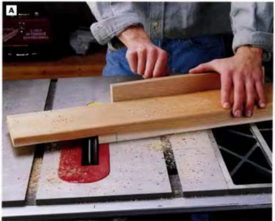
PHOTO A: Cut the half-laps in the seat supports and back supports with a dado-blade set, making multiple overlapping passes. The final pass on each board should be right along the marked cutting line. Set the miter gauge to 65°. Making the half-lap joints prior to cutting the contours of the parts simplifies the layout of the contours.
