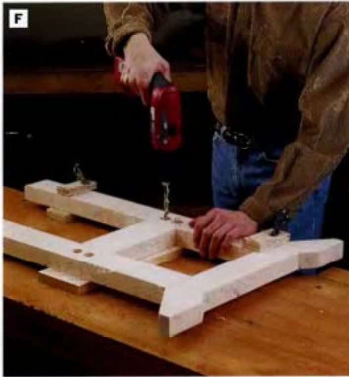
PHOTO F: Drill counterbore holes for the lag screw heads and washers, and drill clearance holes and pilot holes for the shanks of the screws.
