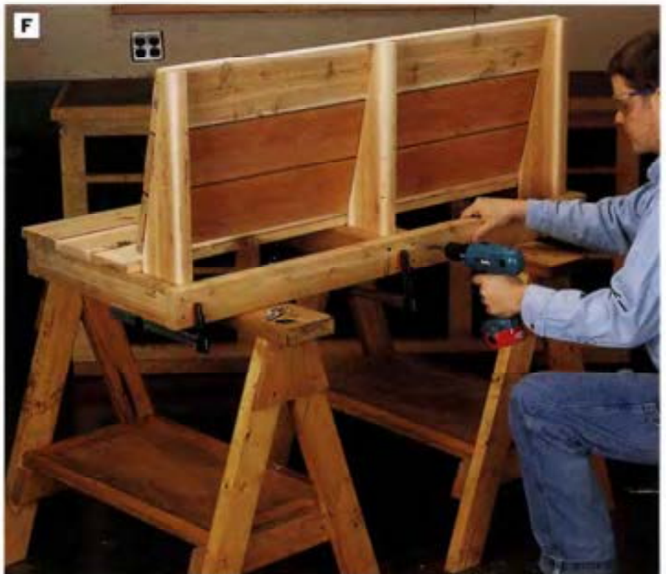
PHOTO F: Fasten the bench back to the seat by slipping the back supports inside the seat frame and between the stretchers, then screwing through the seat frame back and stretchers into the back supports.
