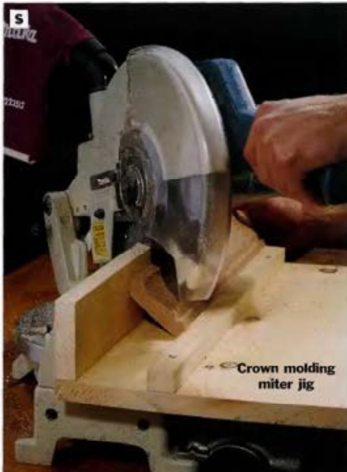
PHOTO S: Miter-cut the ends of the front crown molding strip and the front end of each side strip at 45° to make the crown molding assembly that is attached to the top of the upper cabinet. We used a simple crown molding miter jig to set up the cuts on our power miter saw.
