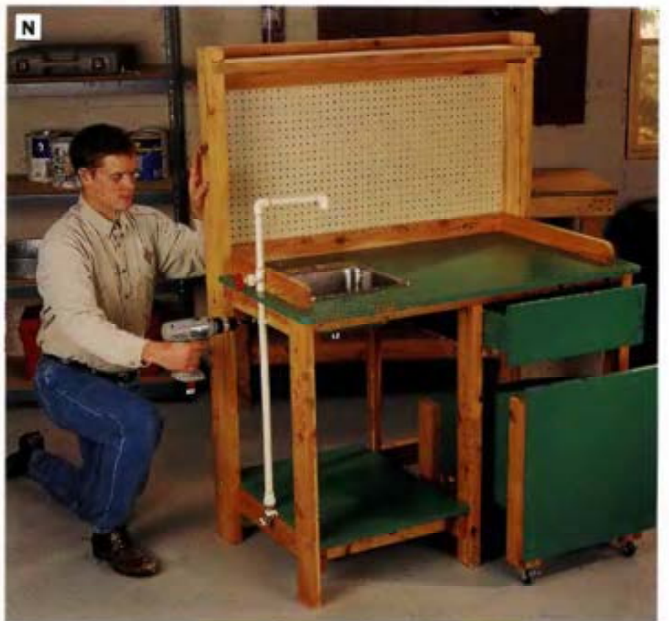
PHOTO N: Use strap clamps to attach the plumbing assembly to the bench.
