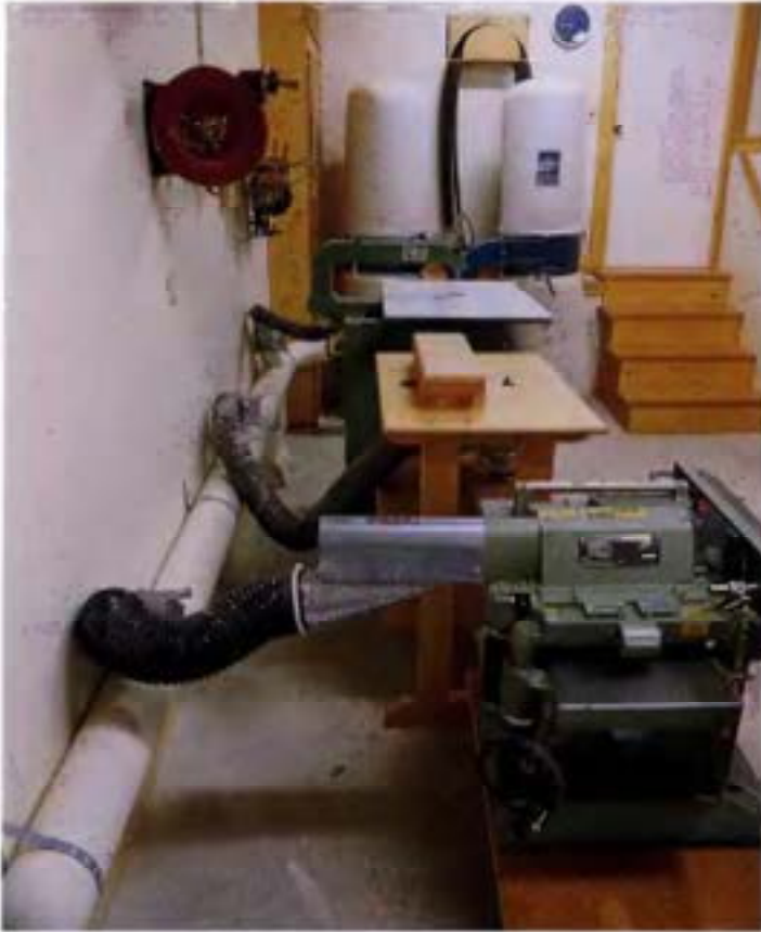
THE TWO-STAGE DUST COLLECTOR in the background of this workshop photo is connected to all of the stationary power tools in the shop with dedicated 4-in. or larger hoses mounted to the walls and positioned to be out of the way when work is taking place.
