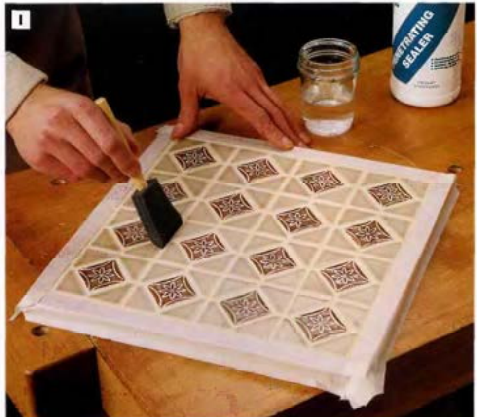
PHOTO I: Seal unglazed tile and grout joints with penetrating sealer. Use a disposable foam brush to apply the sealer. Because a plant stand is likely to be exposed to a considerable amount of moisture, sealer is important to protect the plant stand top and to help inhibit mildew and other forms of discoloration that can affect the grout.
