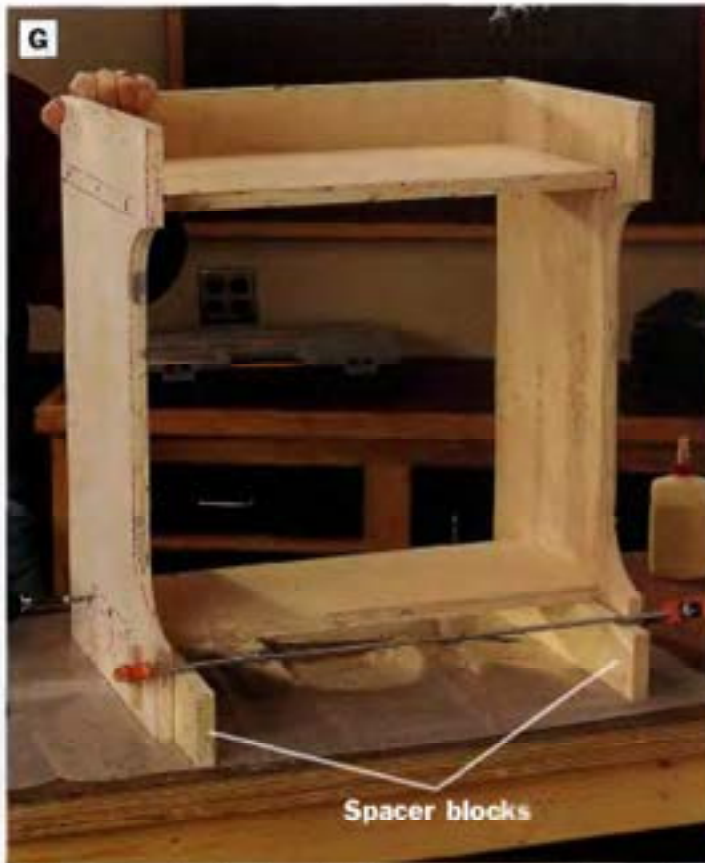
PHOTO G: Install the footrest with glue and screws. Insert a couple of 3/4-in.-wide spacer blocks beneath the footrest to hold it in position temporarily while you screw it in place.
